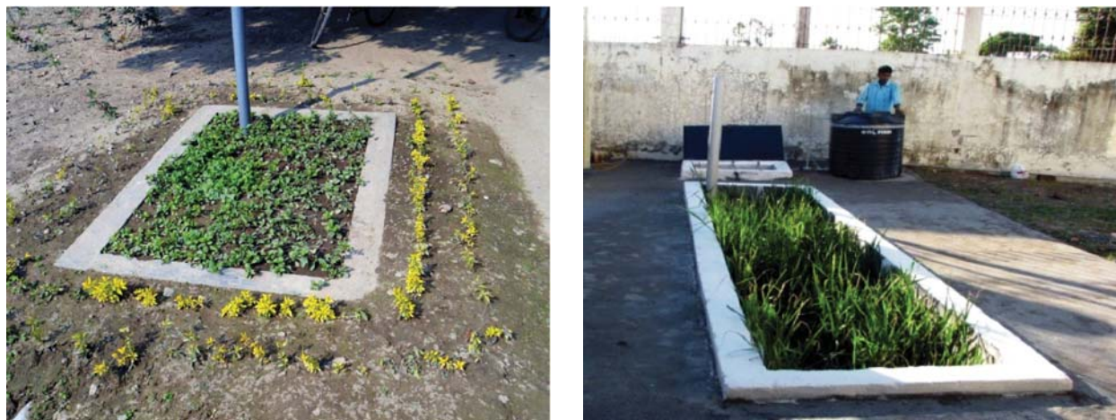
Fig. BioTank cum Reed Bed systems functioning at Defence Research Laboratory, DRDO, Tezpur, Assam
