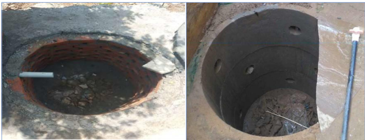
Household Level Leach Pit
