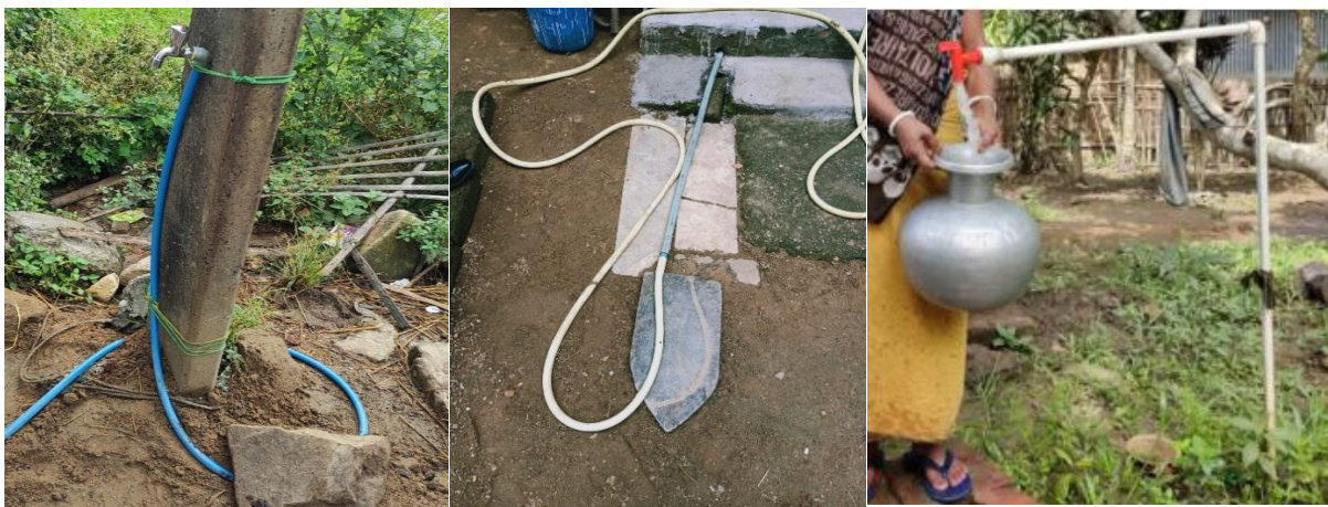
Construction of FHTC – Bad Practice
